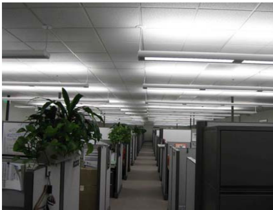
Figure 3: Universal Suspended Lighting System at Test Site
