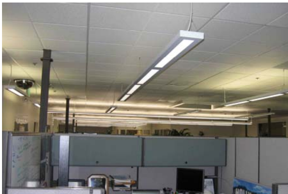
Figure 4: Convia Suspended Lighting System at Test Site
