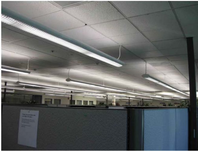
Figure 2: Lutron Suspended Lighting System at Test Site
