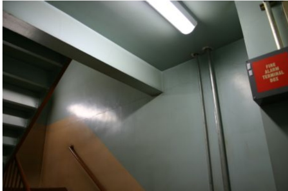
Figure17: Staircase C, light distribution shadow (shadow shows direction of light which reaches mid-floor landing)
