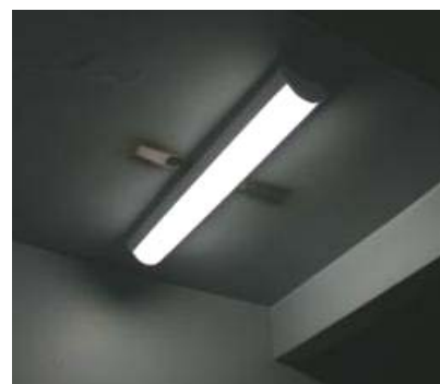
Figure 9: New Occu-smart fixture, and smoke outline of old fixture (mounted perpendicular to the new fixture)
