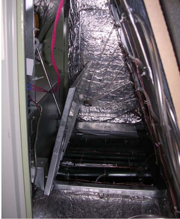
Figure 5: Photo of the economizer damper at the minimum position.
