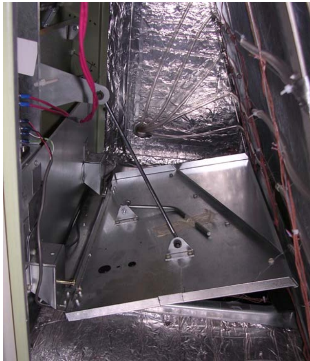
Figure 6: Photo of the economizer damper at an almost fully open position.
